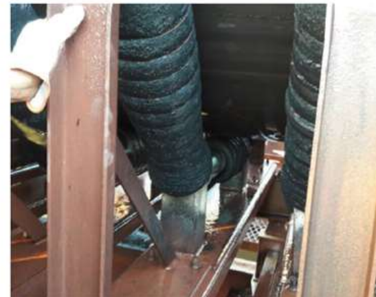
(f) Damaged Rollers
