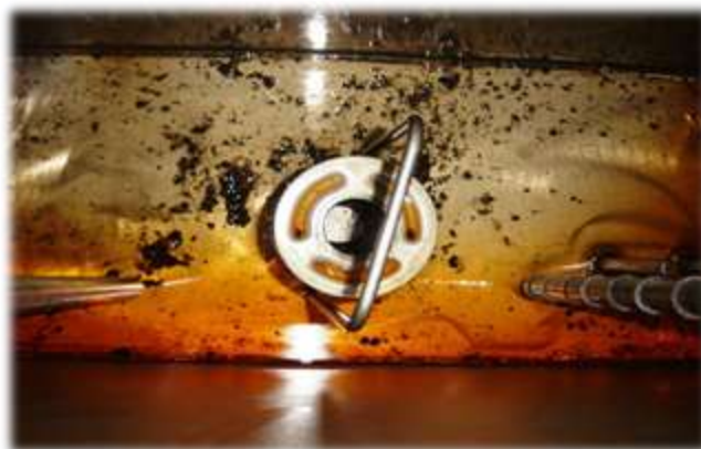
Figure 3. Phosphate ester gels in an EHC reservoir.
